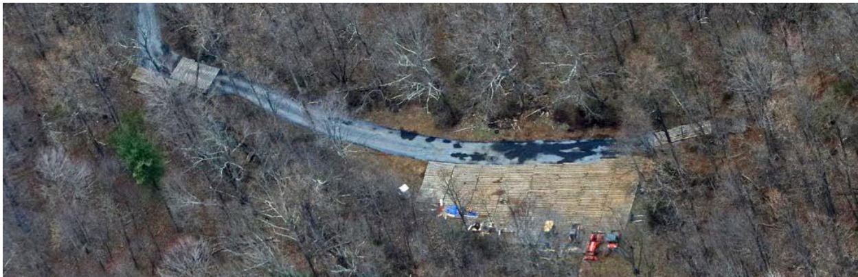
Apparent equipment staging area and new or reconstructed road and bridges observed during Pipeline Air Force surveillance flights. (3/11/18)
